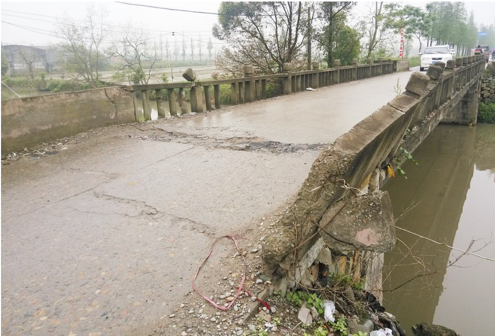
桥梁护栏破损
